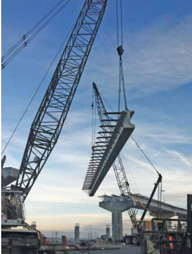
Sundt's crews have finished setting the steel girders on one of the Loop 375 Transmountain West direct connectors and are now in the midst of setting the concrete girders.
