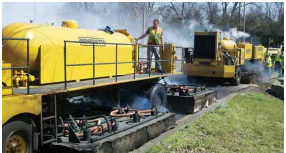
The in-place process eliminated the trucking of more than 30,000 tons of millings and asphalt on one job alone. That equates to more than 2,000 truckloads of resources that will not be driving over other streets and damaging them to get to and from the job.
