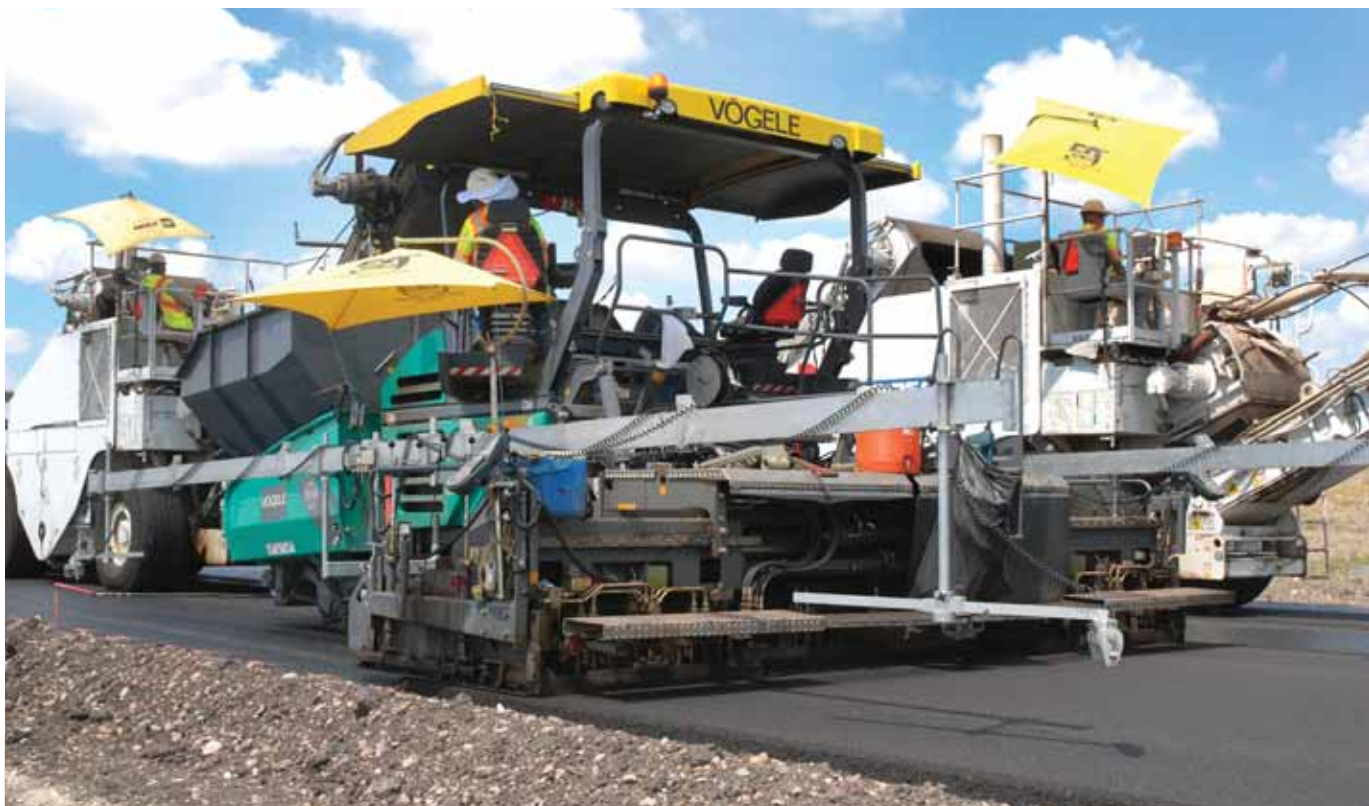
The compaction elements in the screeds were attaining such density that the contractor was able to eliminate three rollers from the train. At the screed, on the coarse Type C wearing course, Industrial Asphalt was obtaining 88 to 90% density.
