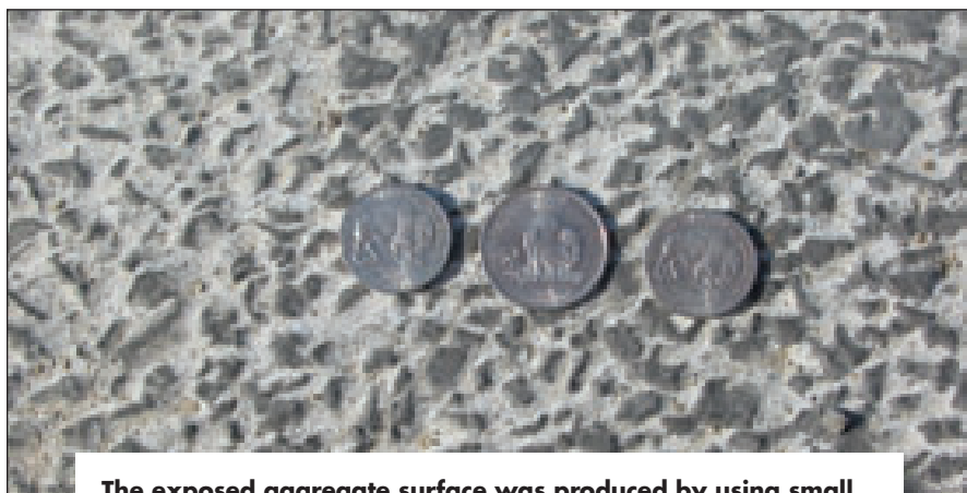
The exposed aggregate surface was produced by using small, wear-resistant rhyolite aggregates. (Photo courtesy of KDOT)
